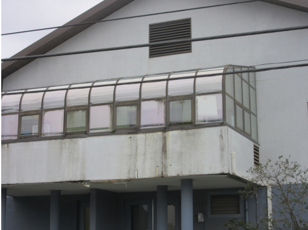
Figure 2-5: Cladding Damage at Long Term Care Wing Exterior Sun Room
