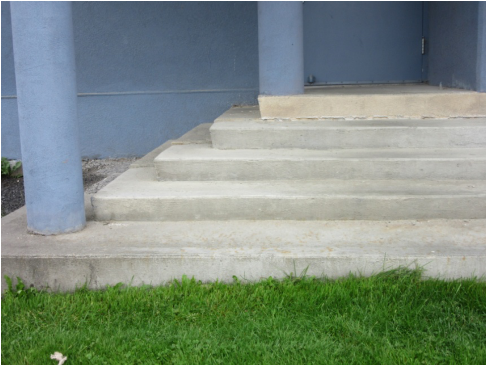
Figure 2-4: Settlement at Long Term Care Wing Exterior Stair
